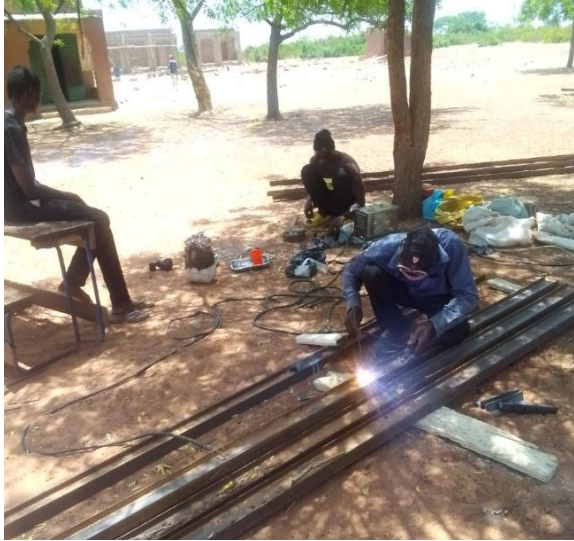
Welding the I-beams for the corrugated metal roof of the school in Tionso, July 2025.
